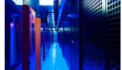
Equinix IBX data center interior (representative photo)
