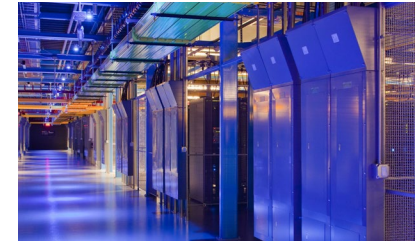
Equinix IBX data center interior (representative photo)
